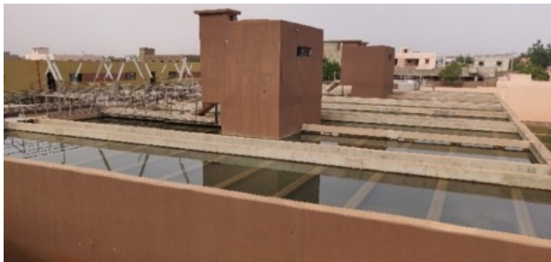
The Kalaba installation
