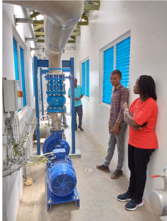
New pumps installed for one of the water supply systems
