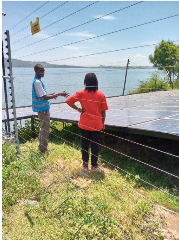
Solar panels fitted to augment energy supply on one of the water supply schemes.
